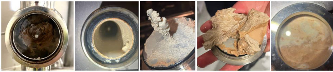
Fig. 11 Initial situation: strong fouling in the UHT with pre-treatment at only 95°C at all critical zones including blocking of components like temperature & pressure sensors
