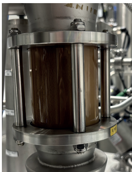
Fig. 10 Sight glass with massive fouling layer [7]
