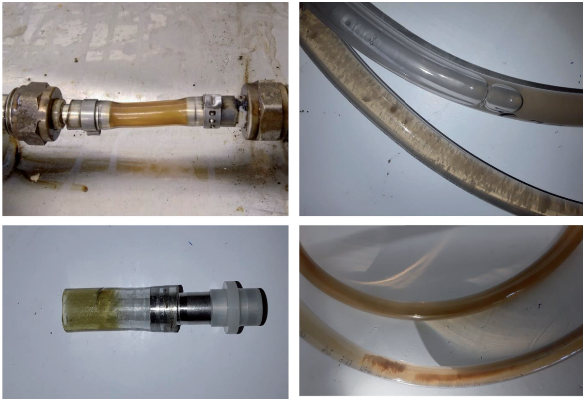
Fig. 1 Exemplary images of spoiled beer transfer tubes showing biofilm formation and fouling on the hose surface with beer contact
