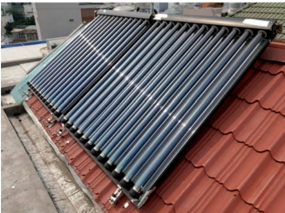
Fig. 8 Picture with 2 CPC Solar Heat panels mounted at the building roof
