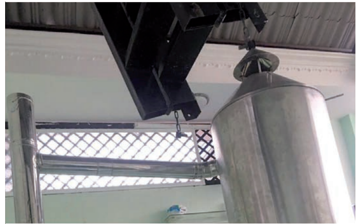
Fig. 9 Picture with Pilot kiln with kiln fan, heating coil and air piping
