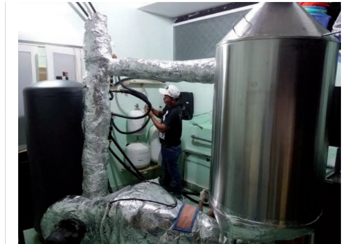
Fig. 11 Picture with pilot kiln connected to the solar circulation, ready for operation incl. insulation
